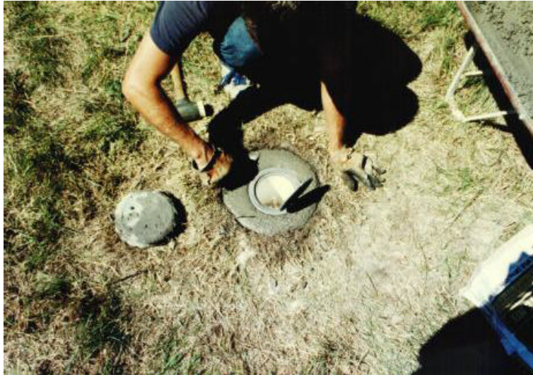
Trowling Smooth Top of Concrete Note, No Concrete on top of Logo Cap
