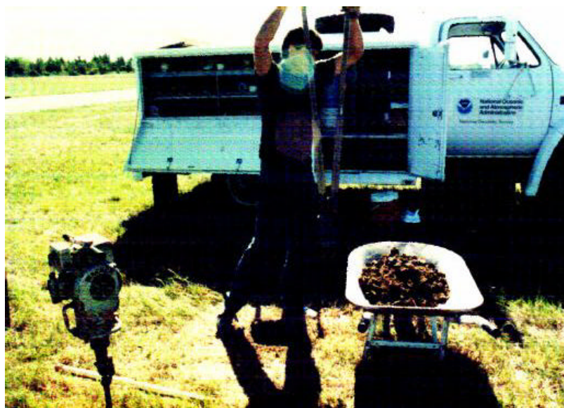
Digging the 43" deep hole; 12"- 14" diameter for the top 22" in depth, and 3"- 6" diameter for the bottom 21" (Note, Dirt removed with a wheelbarrow)
